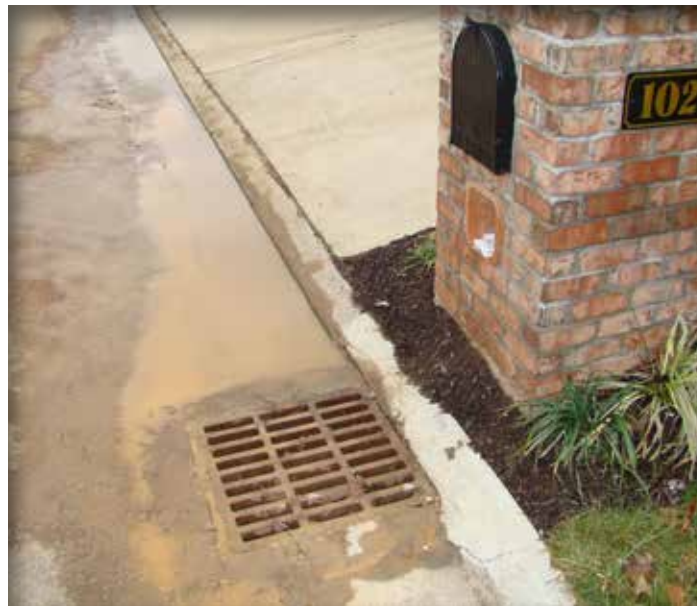
Figure 7-0.1 Jobsite Runoff is identified as an Illicit Discharge
