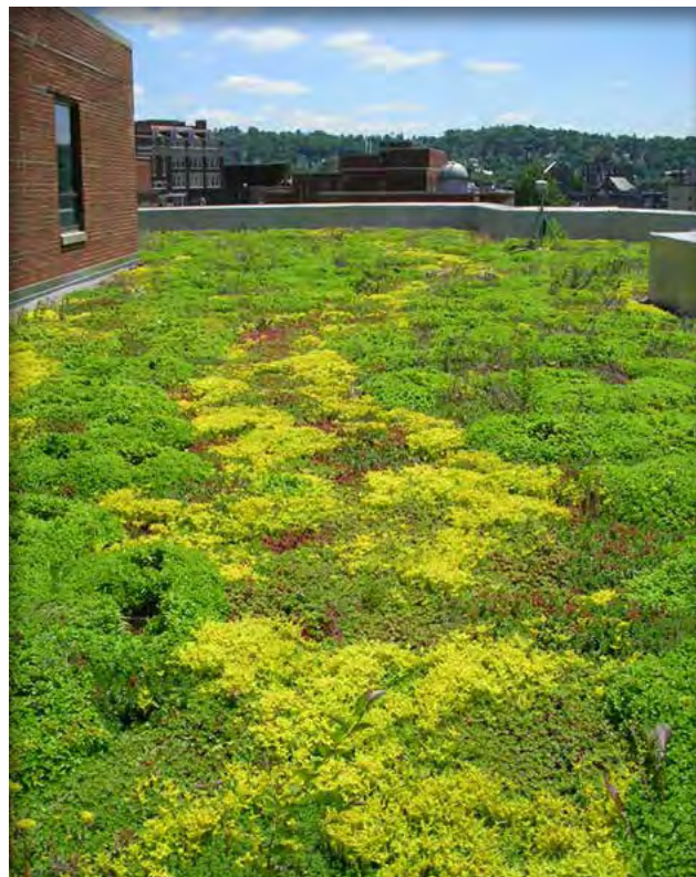
Figure 3-4.14 Green roof at West Virginia University
